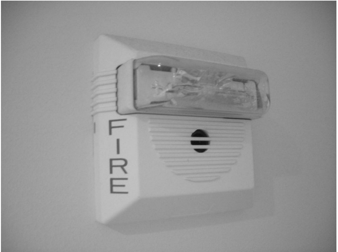
Figure 8-15 Fire alarm annunciator
