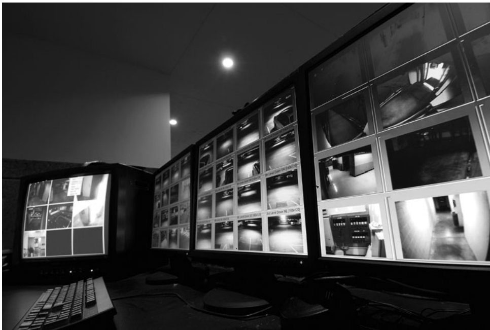
Figure 8-9 Video surveillance monitors
